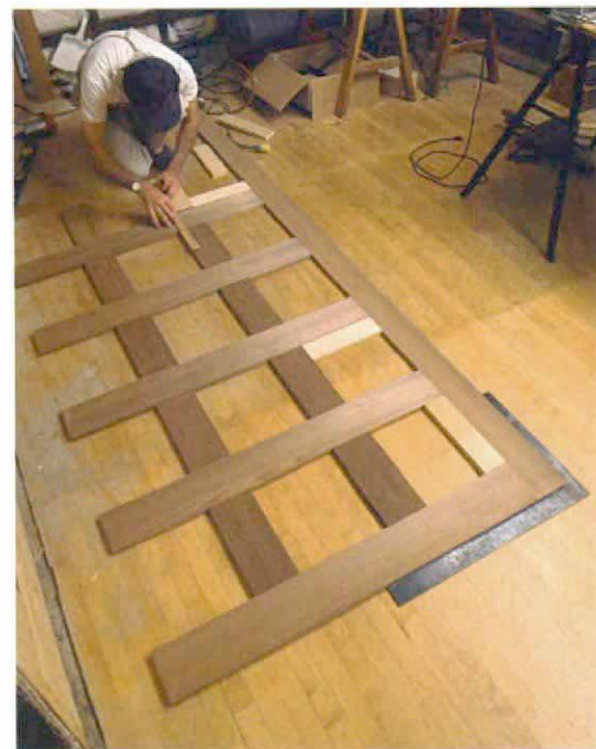
Spacers help to speed an accurate layout. This framework of redwood 1x4s will overlay the wall panels. Here, the author uses spacer blocks cut the same length to mark the positions of upright frame members (photo left). With the uprights in place, the horizontal members are positioned and marked for slotting with a biscuit cutter (photo above).
